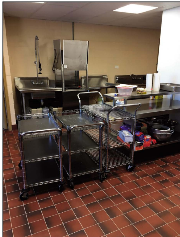
The kitchen at St. Mary’s Parish Center in Brushton was expanded and renovated using funds raised in the ‘It’s Our Church; It’s Our Future’ capital campaign. The previous kitchen did not meet Department of Health standards and could not be used for large events.
